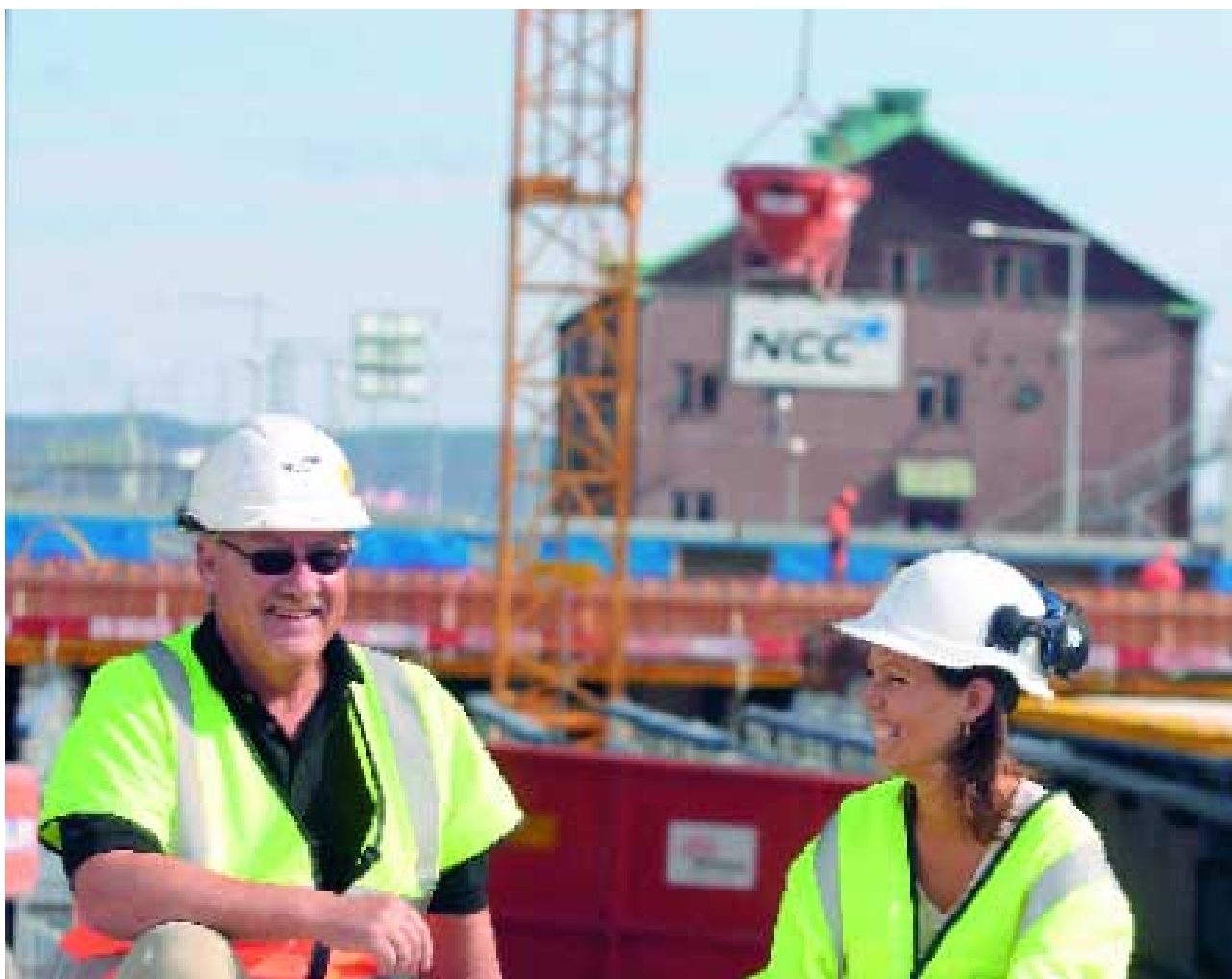
One of the major civil engineering projects in Sweden during 2003 was the ongoing construction of the Göta Tunnel, which is part of the Göta Link designed to improve traffic flows in Gothenburg. During autumn 2003, the project was three months ahead of schedule, thanks to NCC Partnering-based cooperation with the customer. Conny Johansson and Anna Norén are two of NCC's many employees working on the project.
