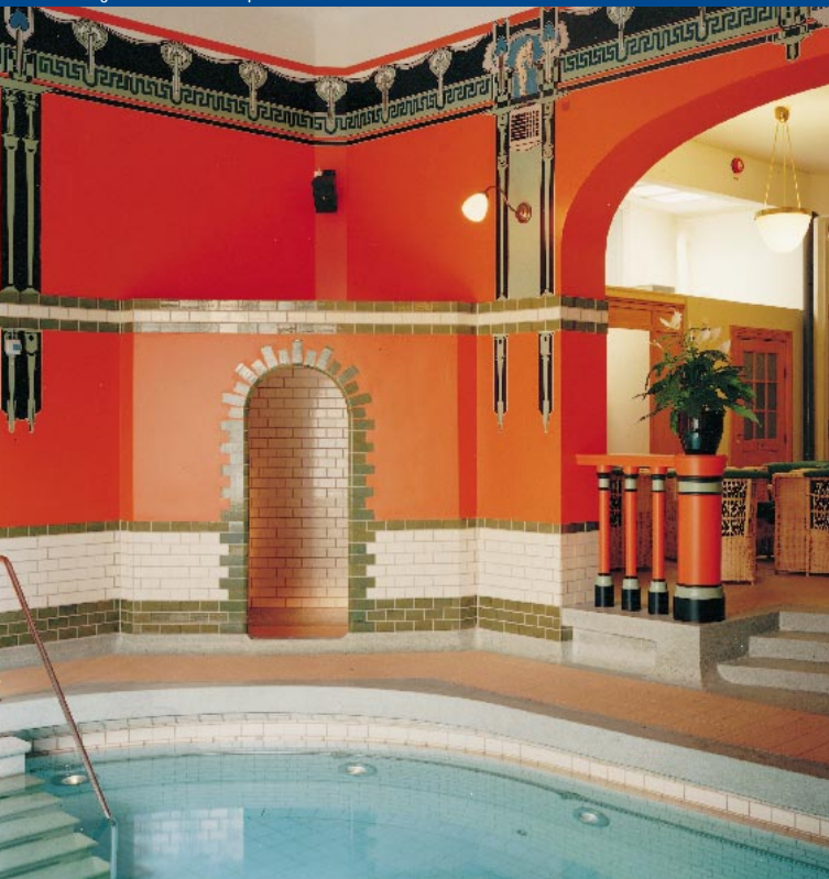
NCC has completed a comprehensive renovation of the Renströmska Baths in Gothenburg. The original building was constructed in the 1870s.
