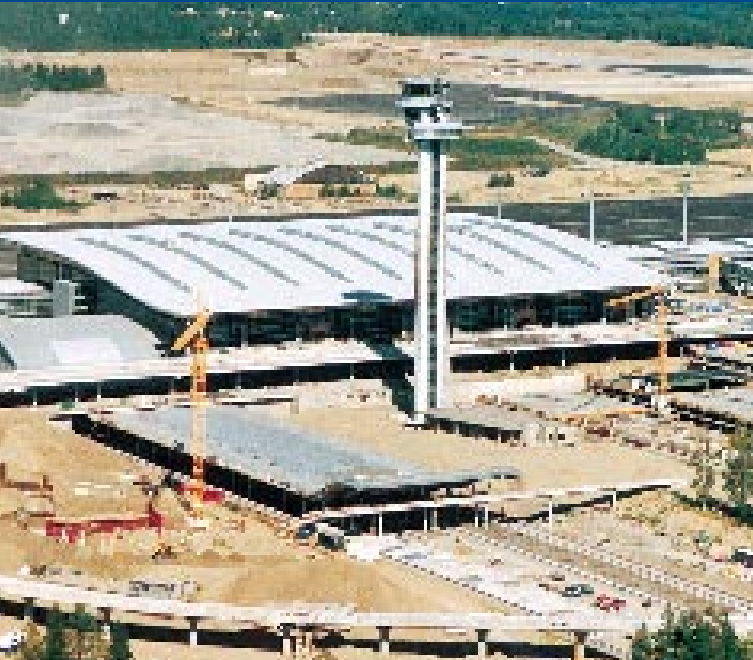
NCC's Norwegian subsidiary NCC Eeg-Henriksen is constructing the terminal building for the new airport in Oslo.
