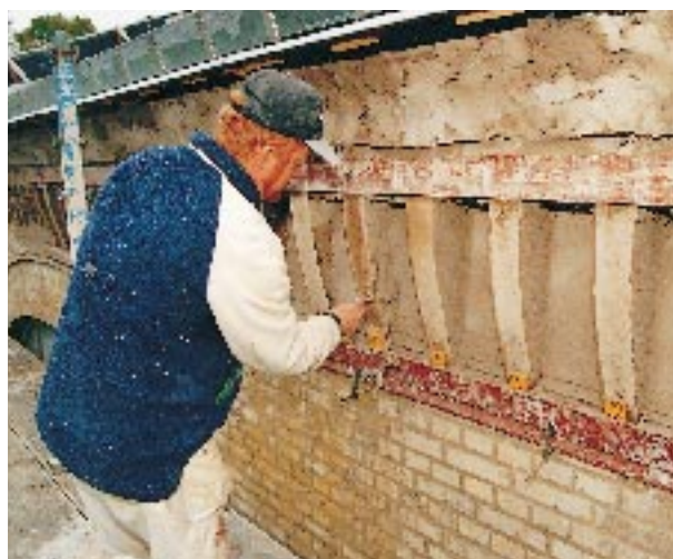
The renovation of Renströmska Badet in Gothenburg using hydraulically applied mortar. More than 2,000 tons of mortar were delivered.
