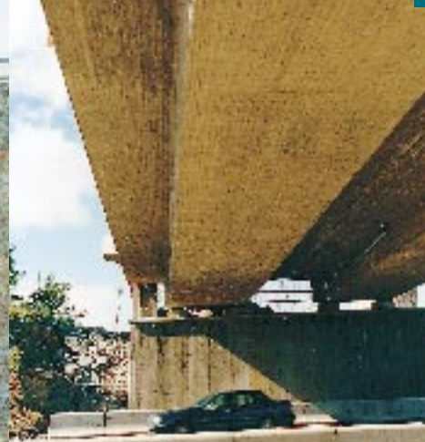
In connection with the Arlanda Link project, this railway bridge over the E4 highway north of Arlanda Airport is being constructed.
