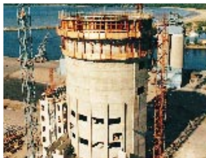
In Halmstad, Sweden, NCC is building an 80-meter-high malthouse with an annual capacity of 75,00 tons of malt.
