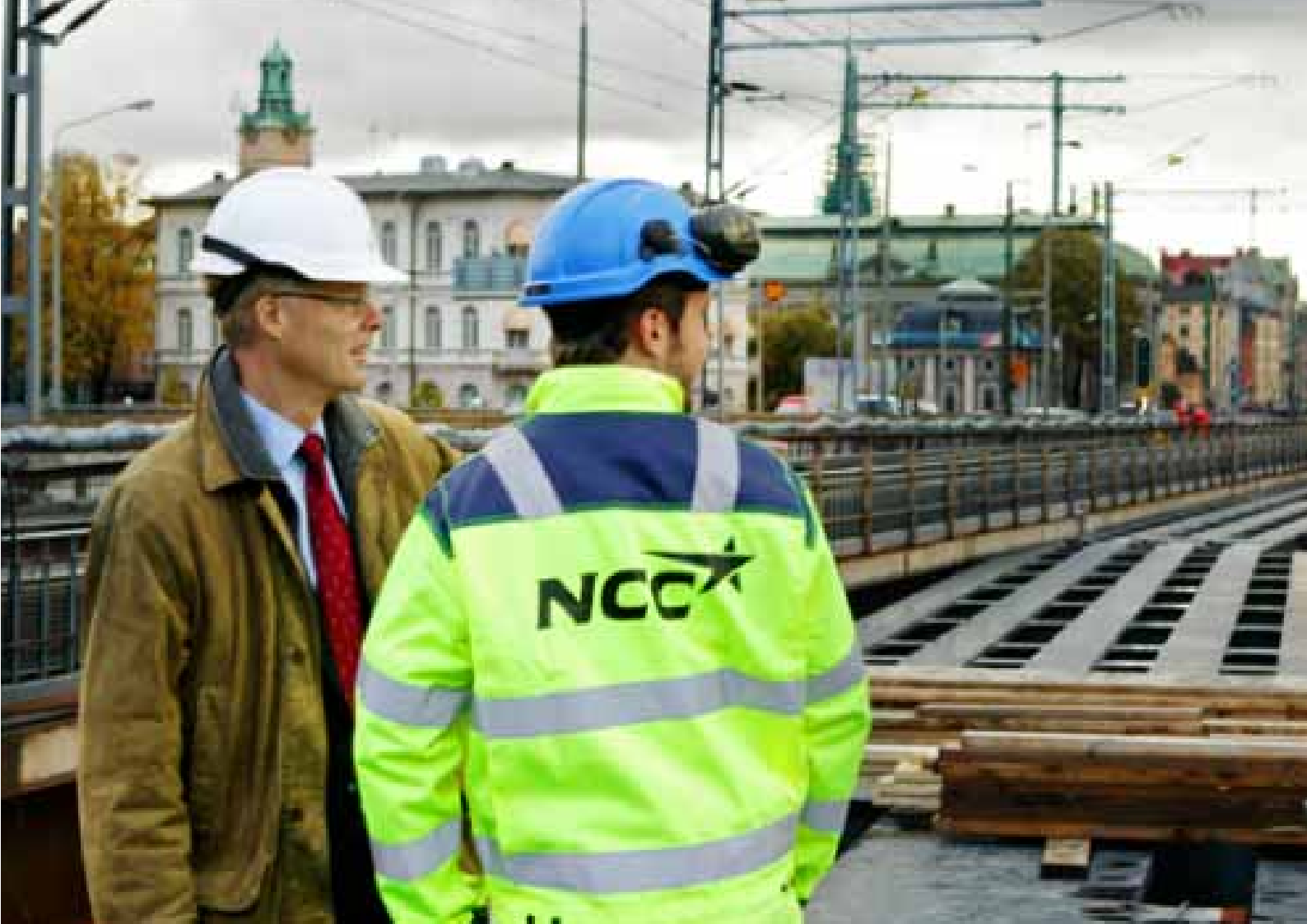
Alf Göransson visiting a construction site at Tegelbacken in central Stockholm, where, among other activities, NCC is rebuilding the signal system, switches and tracks and widening the bridge. He is talking to Johan Rudheden, a trainee within NCC Construction Sweden, Civil Engineering Stockholm/Mälardalen.
